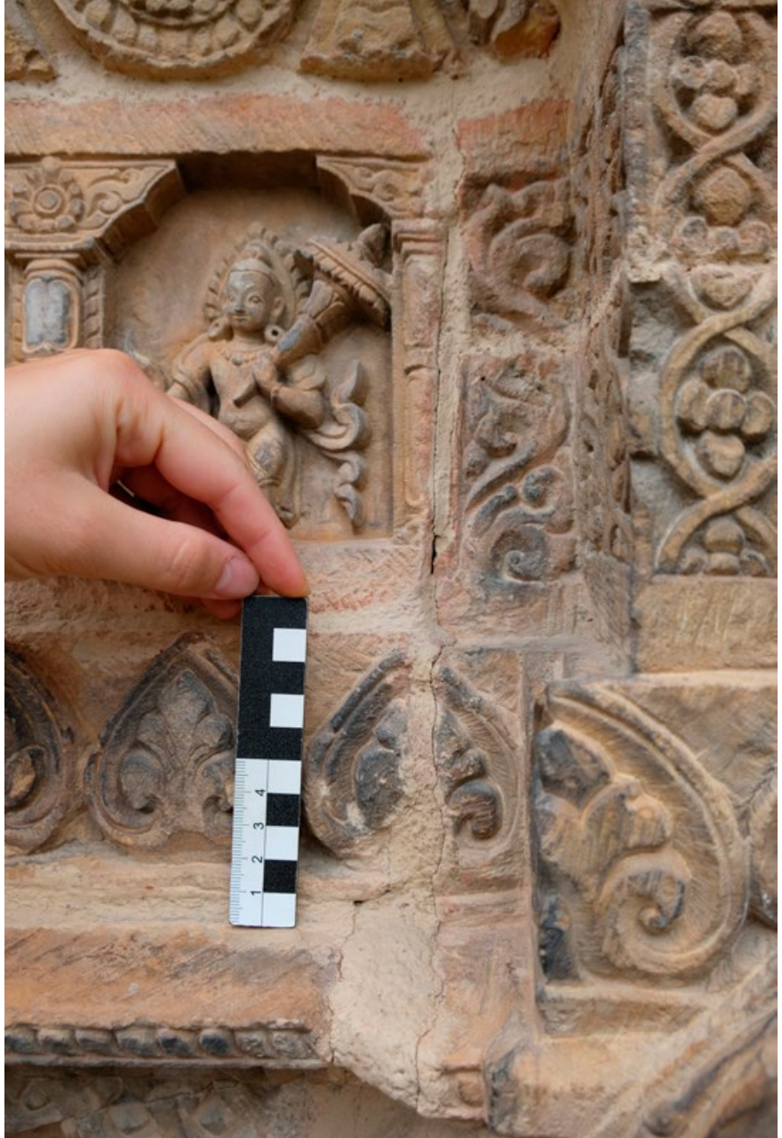
EVALUATION OF PREVIOUS CONSERVATION MEASURES AT BHANDARKHAL TANK PAVILION
